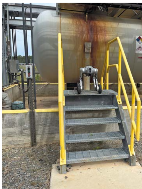
He goes ahead and assesses the situation. If it detects a hazard, employees can see it in real time on a display. The robodog guarding its territory – the Central Plant.
